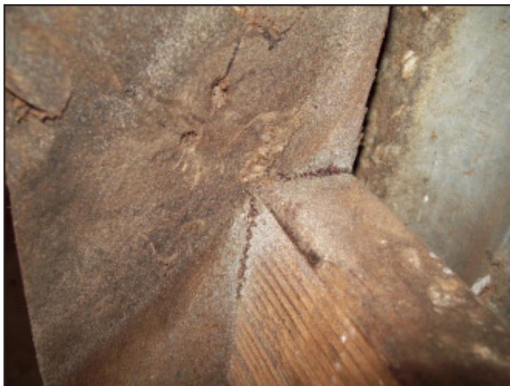
Red Mite are easily seen after there feeding and are found in cracks in all parts of the Fowl Coop.
